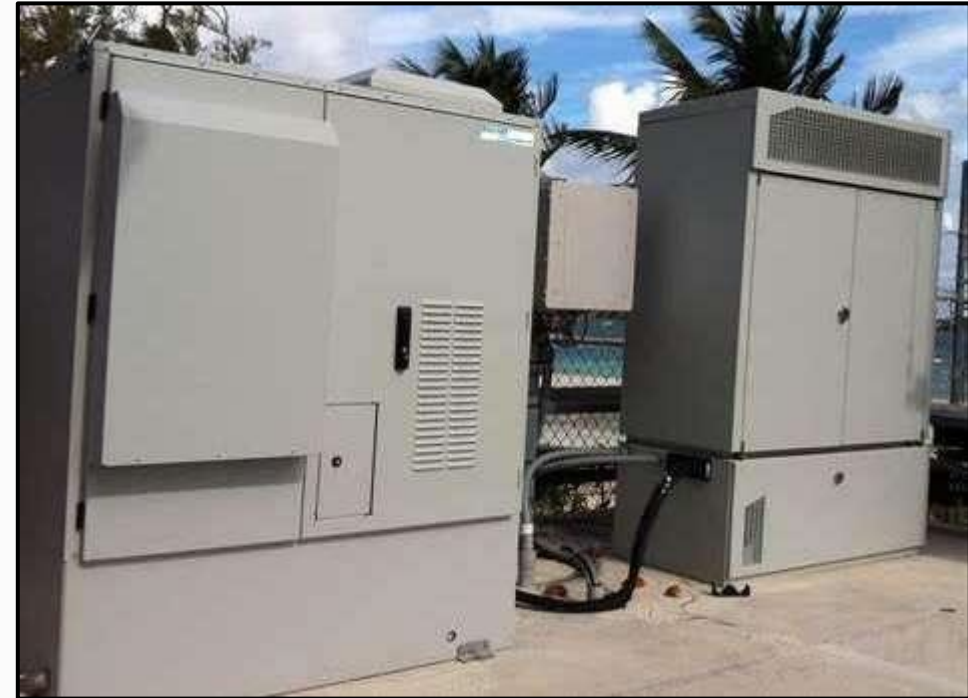
5G Signal Tower Off grid power
