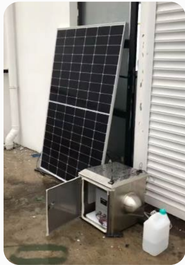
Long-lasting independent power solution Providing power regardless of weather conditions
